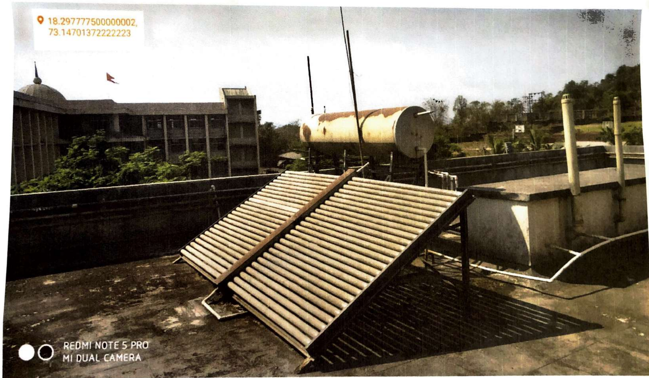
Solar water Heater
