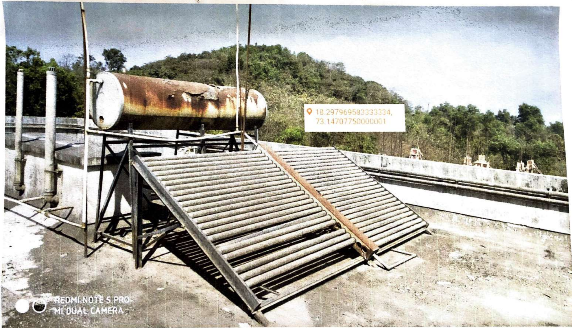
Solar water Heater
