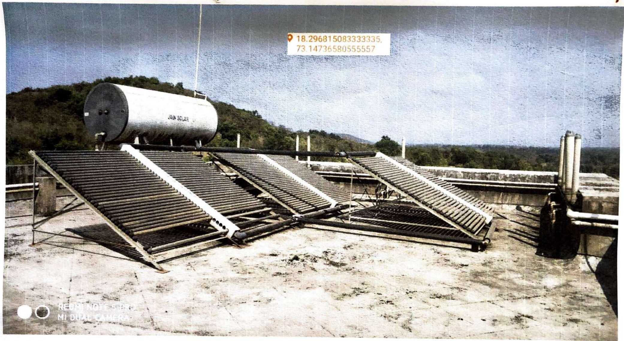
Solar water Heater
